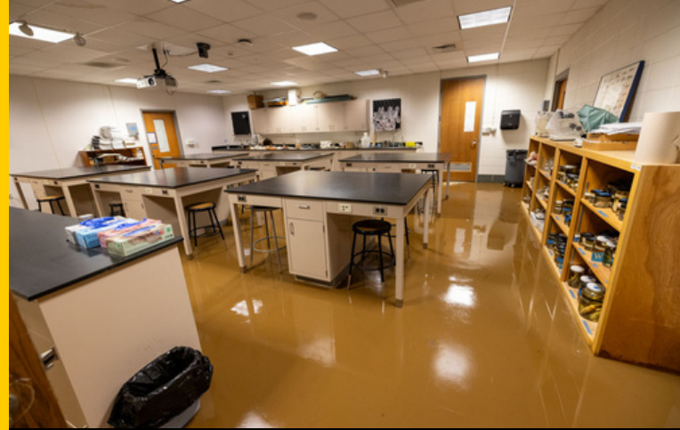
Flooding in Rankin Science West Basement Lab picture by Chase Reynolds
